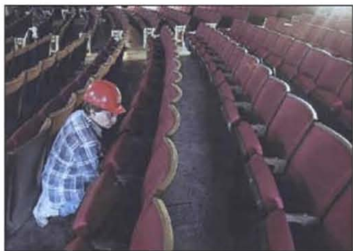
Construction worker Gary Mesko puts bolts in the new seats in the auditorium of the Civic Theatre.
